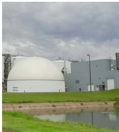
At Cavendish Farms on Prince Edward Island, digesters break down potato waste, producing biogas that fuels the boilers in the company's nearby French fry processing facility. (Image: Pat Martel/CBC)
